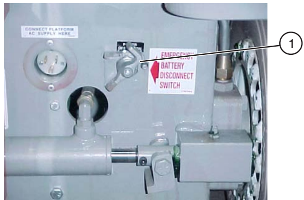
Figure 2-2. Emergency Battery Disconnect Switch
