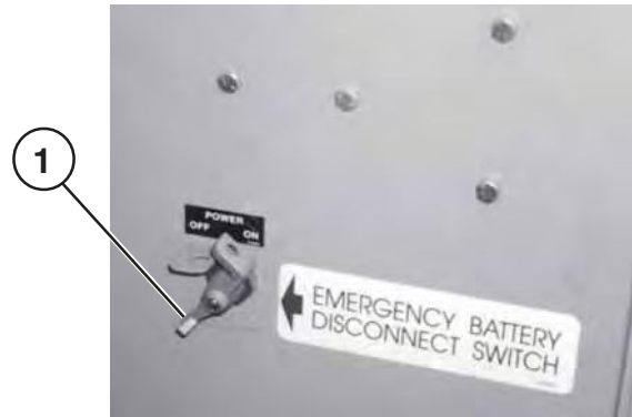
Figure 2-2. Emergency Battery Disconnect Switch
